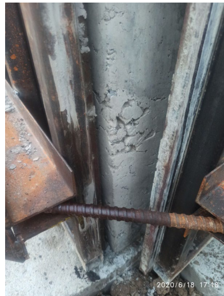
Figure 7: Quality defects in column casting
